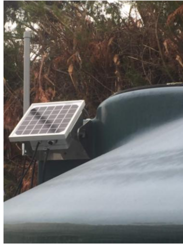
Figure 2: Tank Level Meter with solar charging
